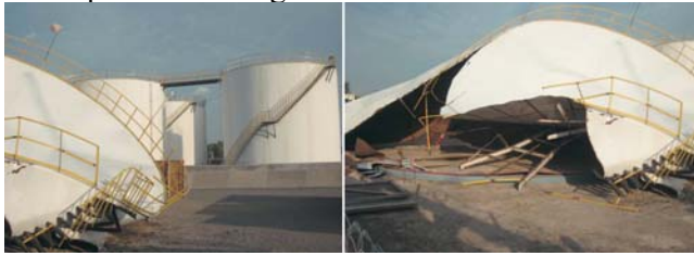
Figure 2. Collapsed water and nearby liquid fuels tanks. Figure 3. Collapsed water tank.
