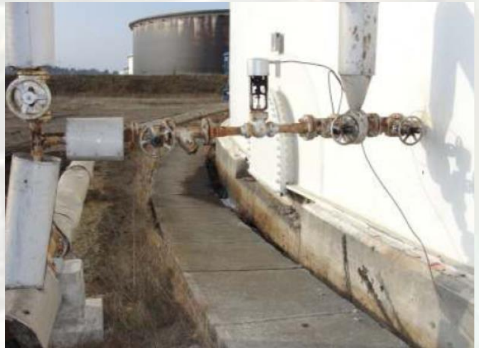
Lateral spreading and soil liquefaction
