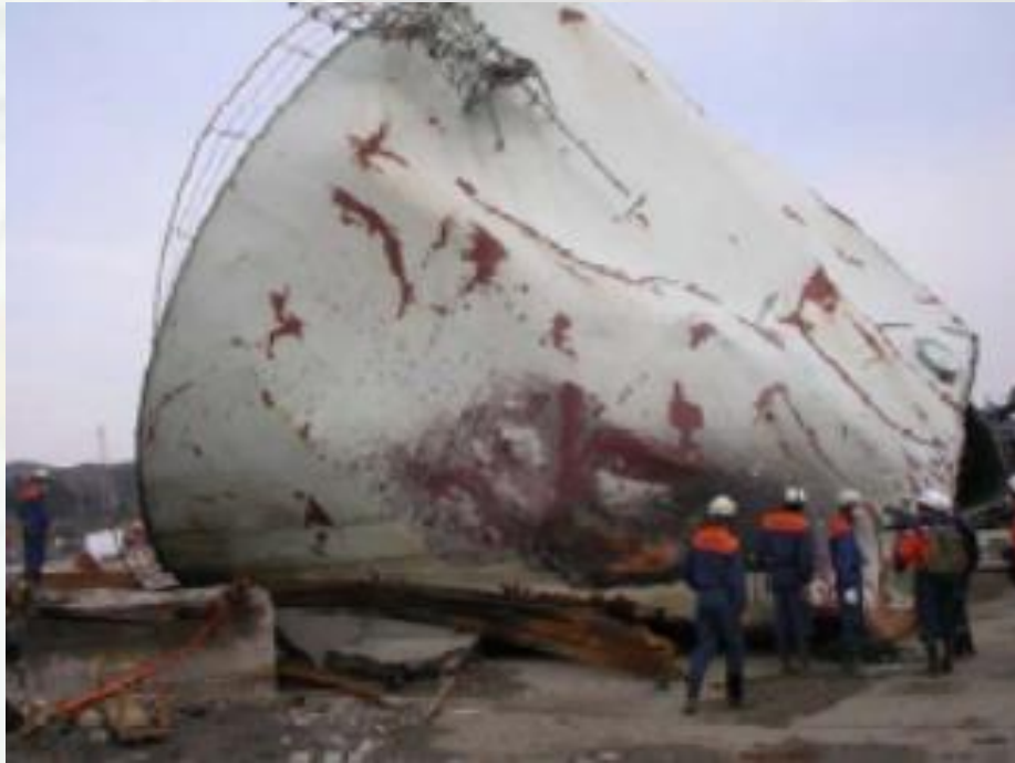
Collapsed by the Tsunami
