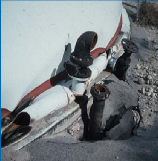
Rupture of Pipes
