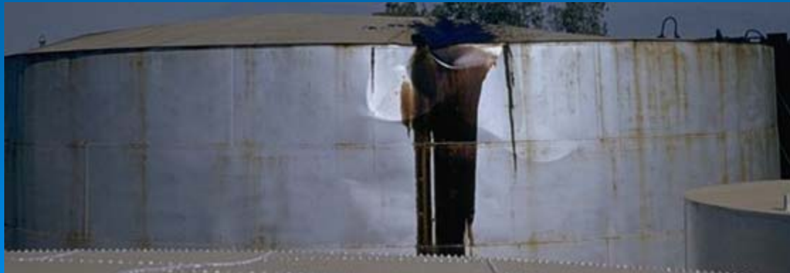
Failures in Joints Wall – Roof
